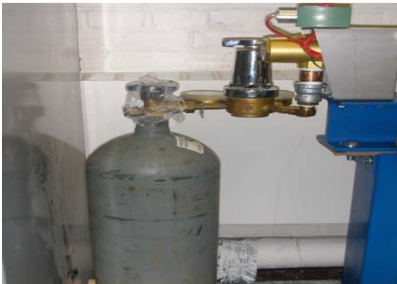
Fig7. Gas tank, solenoid valve and pressure regulator.
