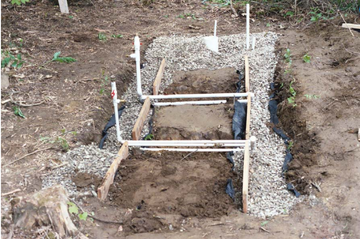
Figure. 3 A photo of the complete test pit with PVC pipe for reference targets and large diameter pipe at far end connected to the drainage system and pump.
