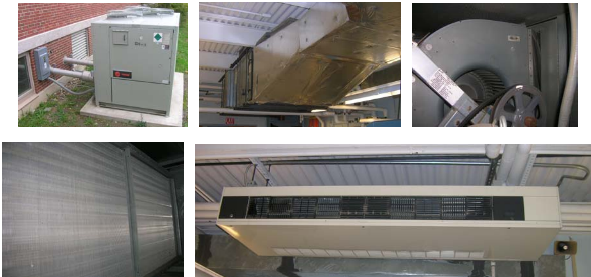
Figure 3 – System Components Clockwise from top left: Chiller, Main Air Handler, Main Fan, Cooling Coil, and Individual Room Cooler
